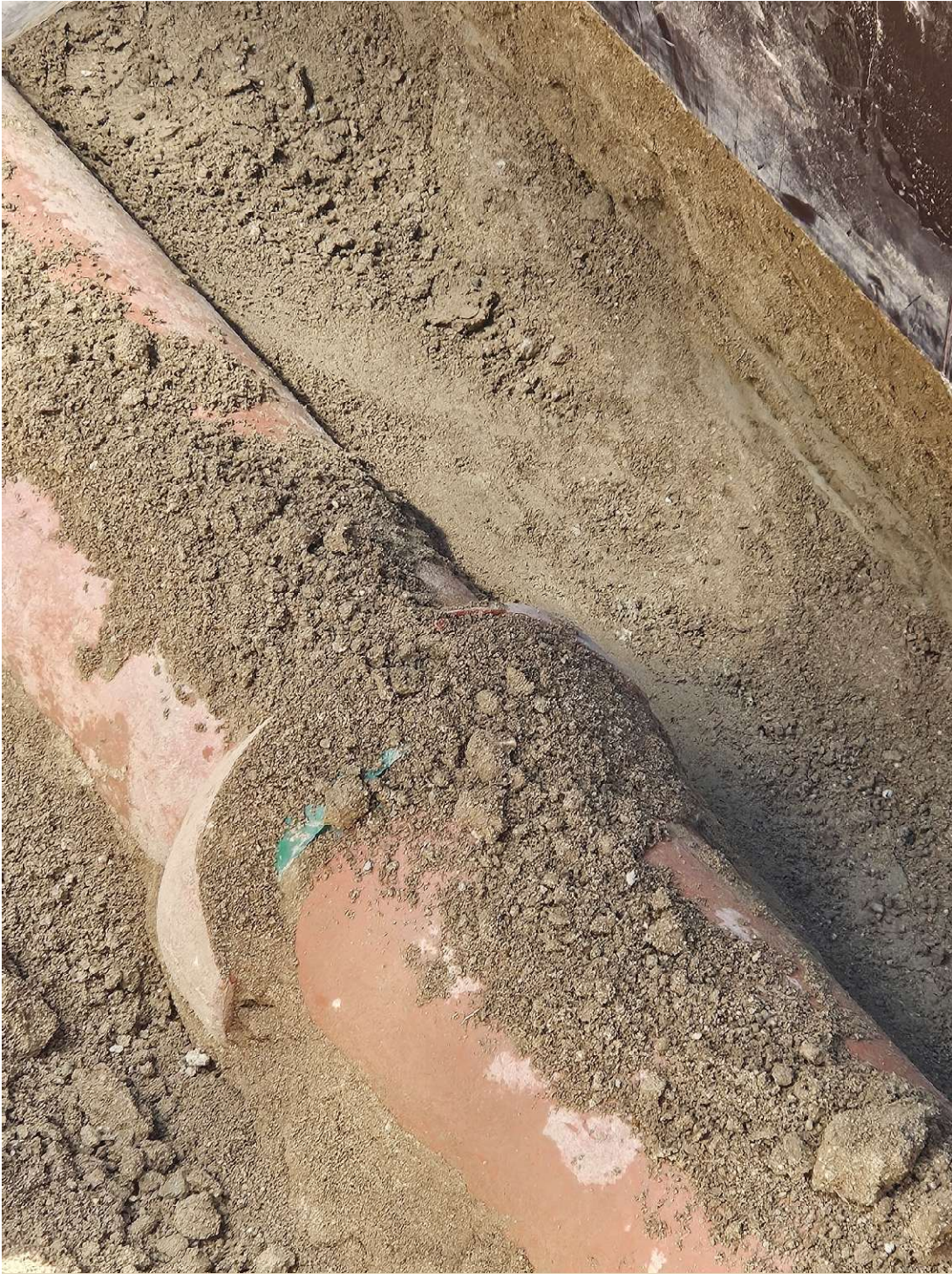
Diamond st VCP sewer pipe with fractured bell
