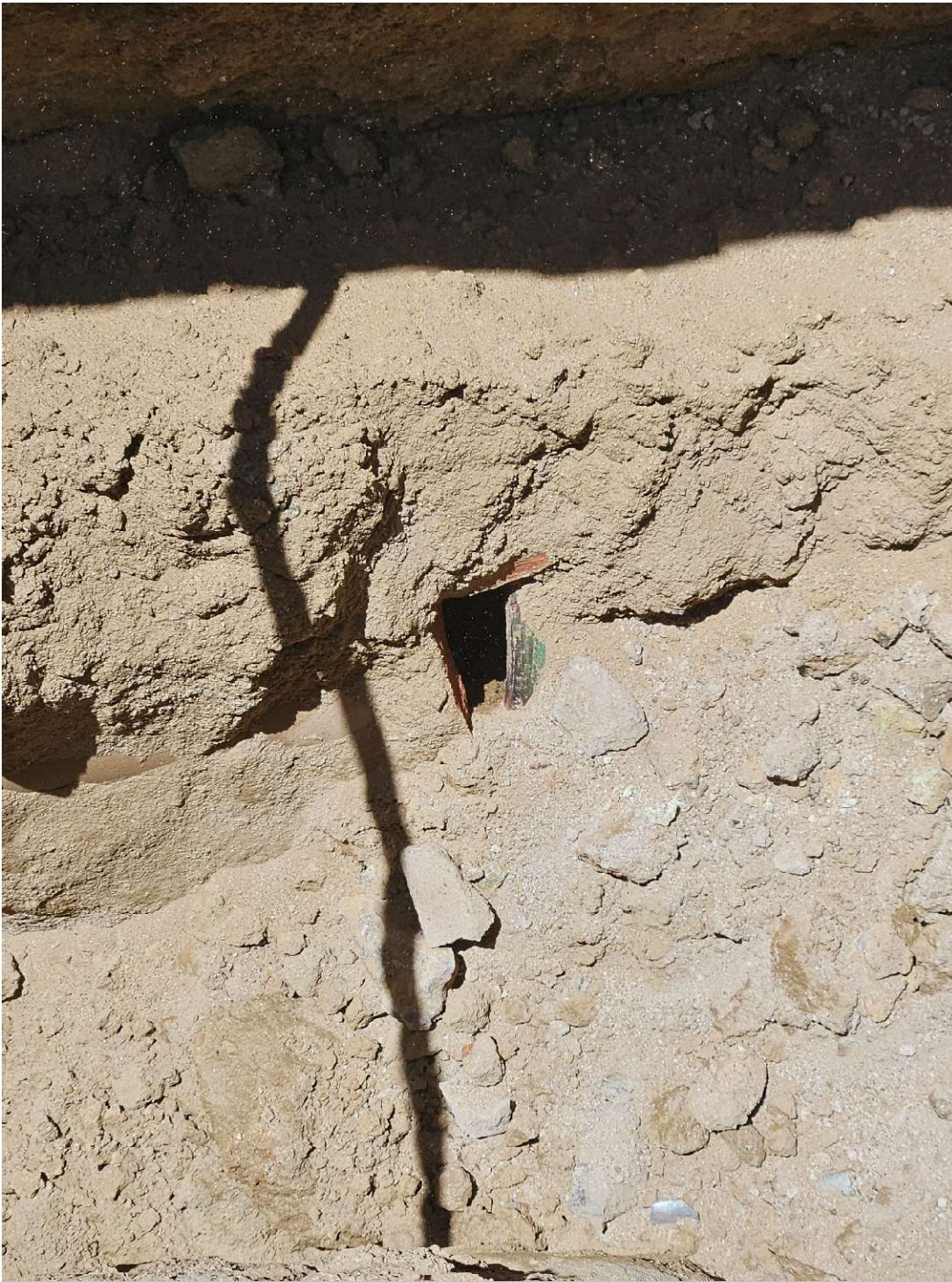
Sewer pipe separation and belly/sag visible on the diamond st sewer line.
