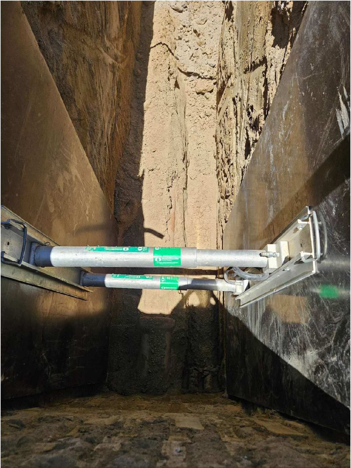
Diamond st sewer line replacement project. VCP visible at the bottom of the trench with shoring jacks.
