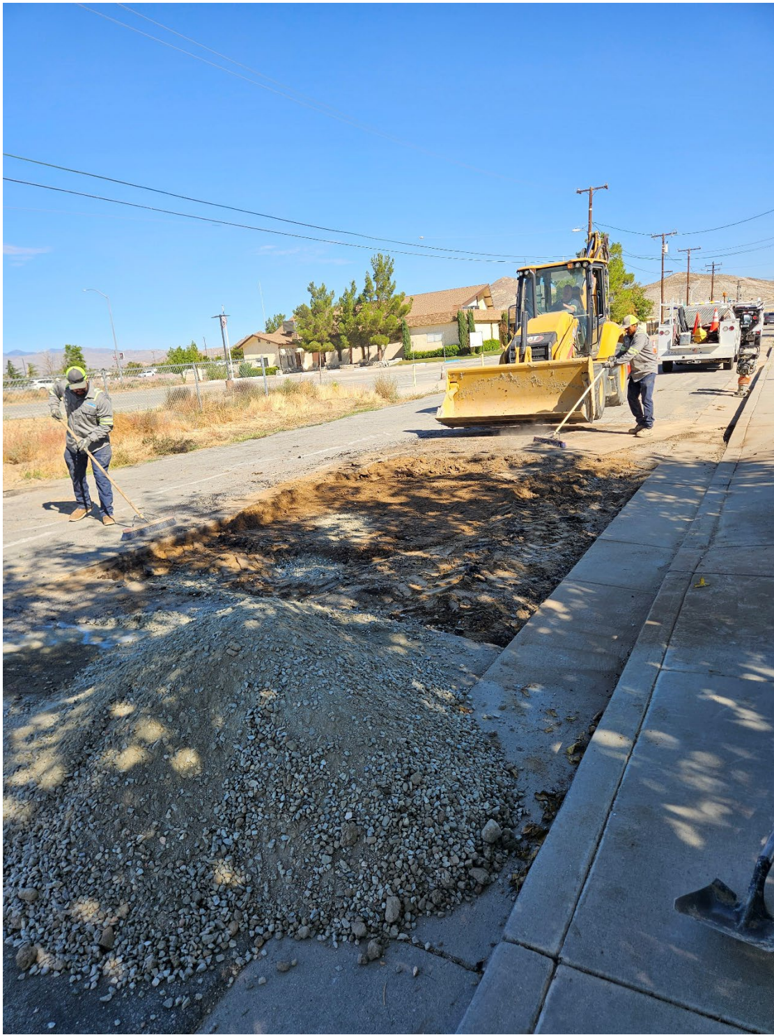
A large service leak on C street caused a sink hole and destroyed asphalt.
